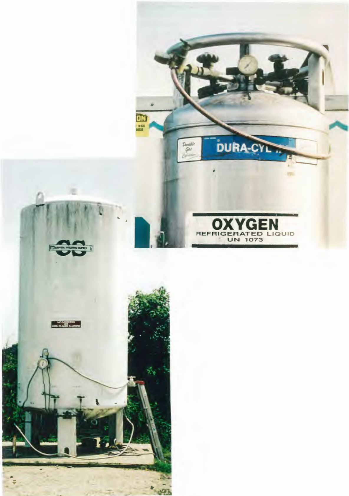
Figure 13 (Above) Liquid oxygen tank fitted to live fish transport truck. (Below) Liquid oxygen storage tank.
