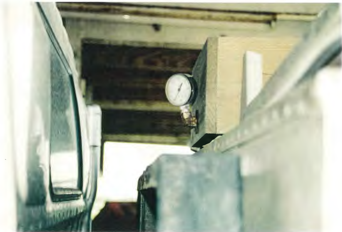
Figure 14 (Above) Controls for live fish transport tank, including: individual flow controls for each air diffuser, oxygen supply system pressure gauge, individual switches for agitators. Note agitator held in place with 'De-Sta-Co' latches, plugged into waterproof 12V power supply. (Below) Oxygen supply system pressure gauge, located to be visible in driver's rear view mirror.
