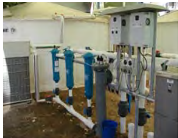
Figure 2. Primary water treatment for "new" incoming water including bag filtration, UV sterilizers, heat exchanger
