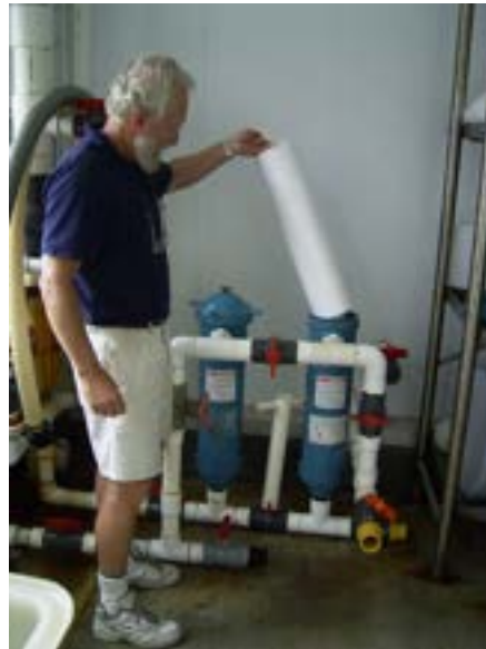
Hatchery seawater filters
