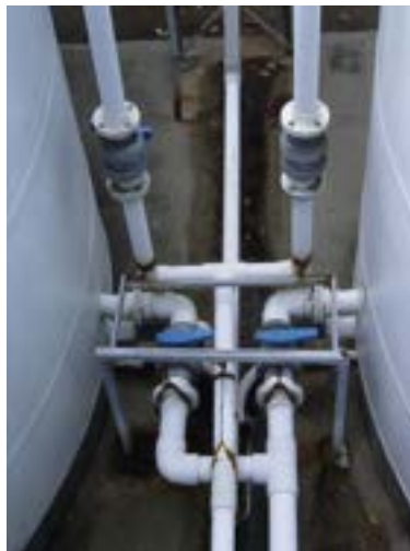
Water storage tank plumbing
