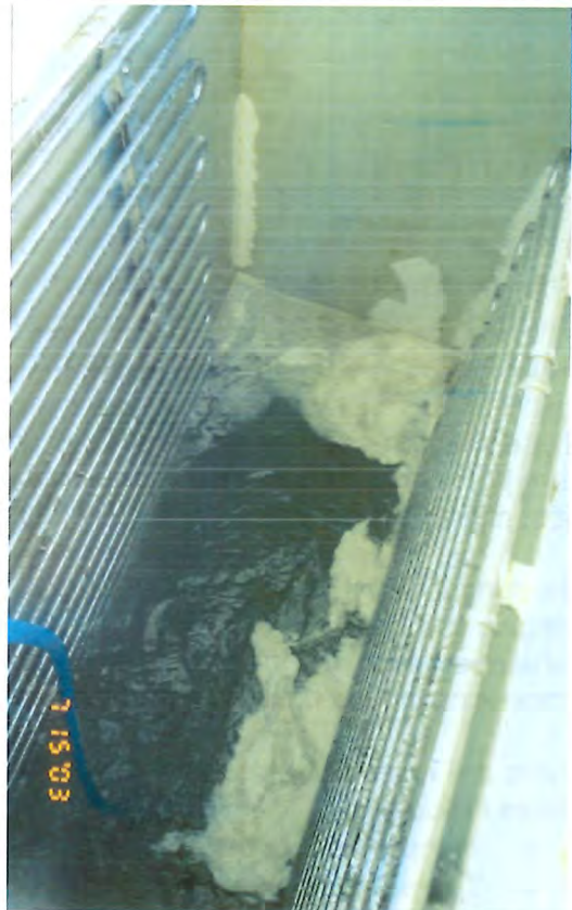
RSW TANK WITH EXPOSED COILS
