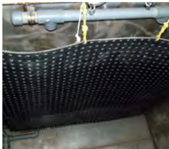
Rubber mats on the wall of the RSW tank protect fish. The holes are to ensure that circulation is even.
