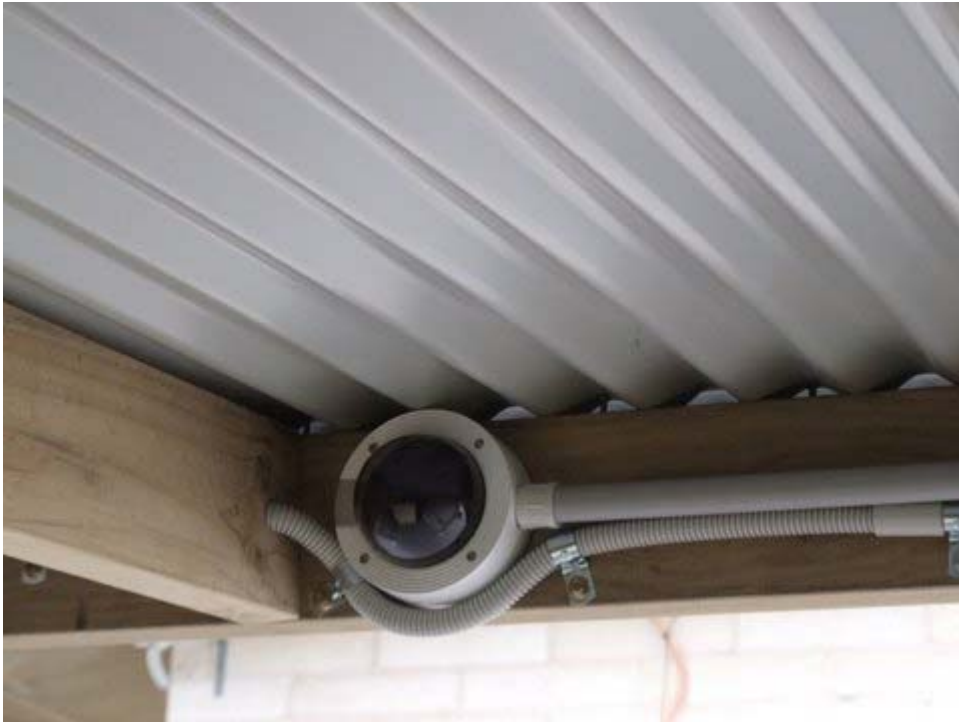
Figure 7 – Cameras Covering General Area
