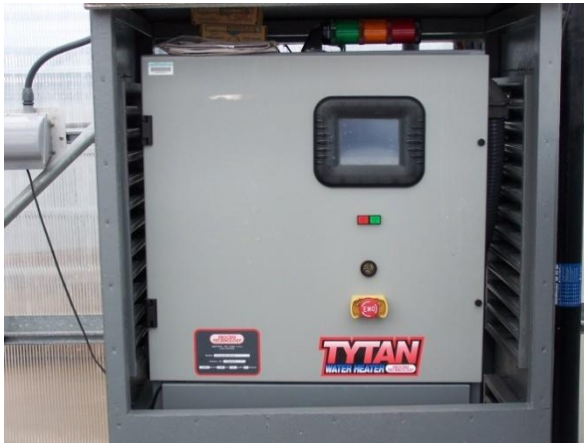
Electric field water heater
