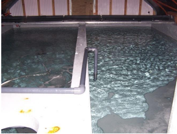
'Clean' water storage tank
