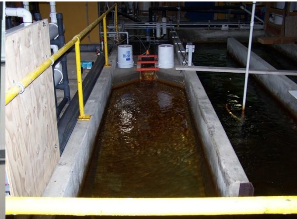
Chlorination channel in quarantine area
