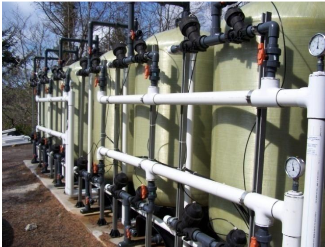
New sand filters
