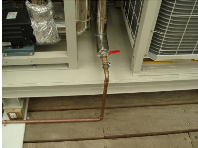
Figure 4. Water intake valve
