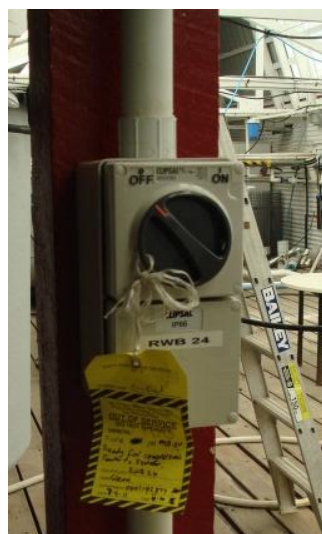
Figure 3. 3 phase power switch
