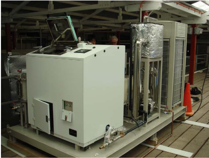
Figure 1: Biolite Dryer installed at Australian Centre for Applied Aquaculture Research
