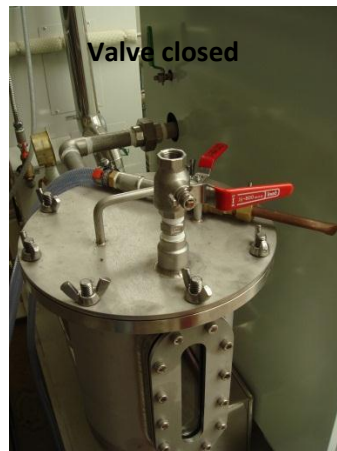
Figure 13. Reclaim pot vacuum valve in the closed position
