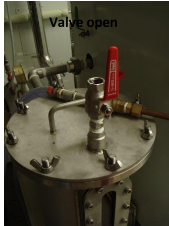
Figure 14. Reclaim pot vacuum valve in the open position
