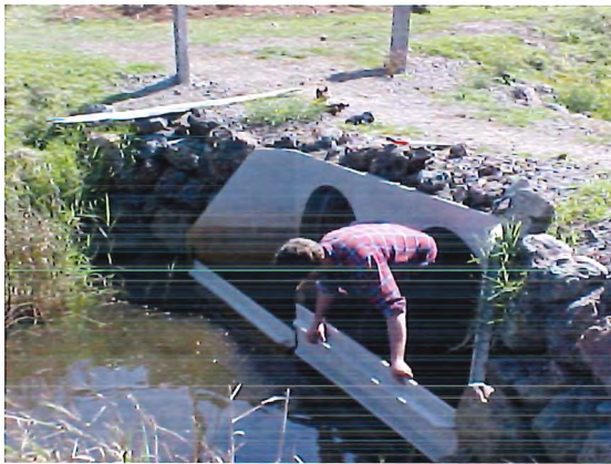
Adjustable drop-boards used for water retention.
