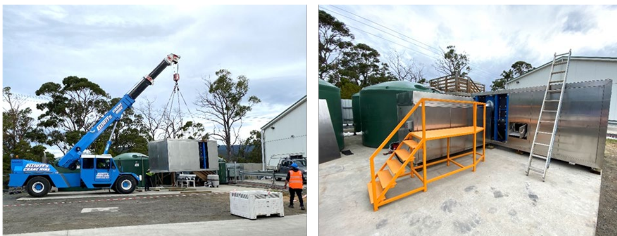
Figure 1. Sea urchin waste processing facility installation at True South Seafoods (Electrona, Tasmania) in May 2021
